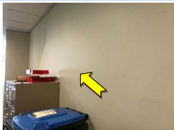
Photo 60. Interior, level 1, walls – suspected lead-containing cream upper paint systems.
