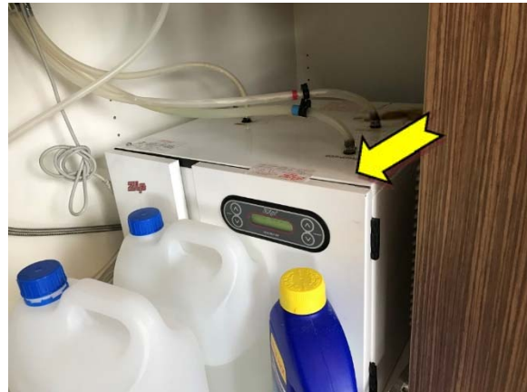
Photo 46. Interior, level 2, staffroom, hot water heater – suspected SMF internal insulation material.
