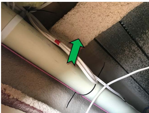
Photo 5. Interior, level 3, meeting room 2, ceiling space, to support beams – non asbestos-containing insulation.
