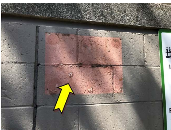
Photo 59. Exterior, throughout, street level, brick wall – suspected lead-containing red lower paint system.
