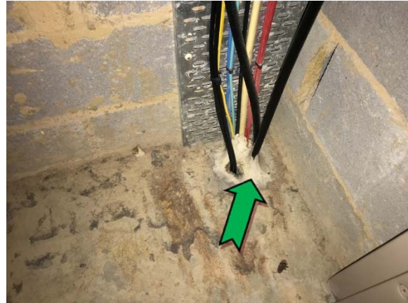
Photo 8. Interior, level 3, comms room, floor, to penetration point – assumed non asbestos-containing mastic sealant.
