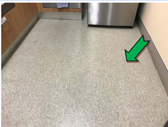
Photo 17. Interior, level 2, main office, kitchen, floor coverings – suspected non asbestos-containing sheet vinyl.
