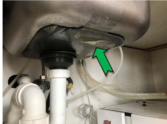
Photo 14. Interior, level 2, staff room, under sink, sink pad – non asbestos-containing bituminous material.
