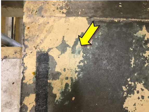
Photo 61. Interior, level 1, floor – suspected lead-containing yellow upper and green lower coloured paint systems.
