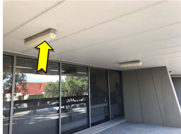
Photo 56. Exterior, throughout, single tubed fluorescent light fittings – suspected PCB-containing capacitors.
