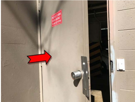
Photo 1. Exterior, north-east elevation, adjacent garage roller door, fire door – suspected asbestos-containing fire door core.
