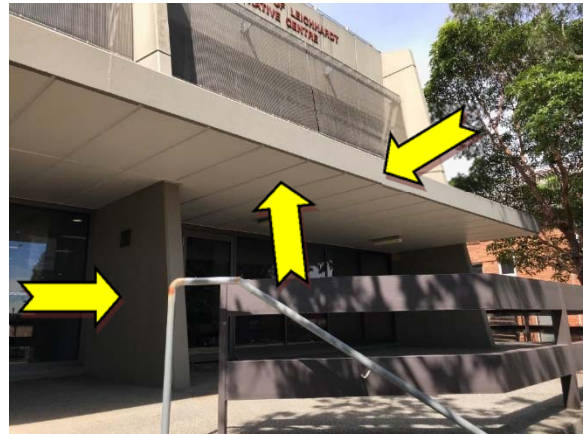
Photo 58. Exterior, throughout – suspected lead-containing white, light and dark brown upper coloured paint systems.
