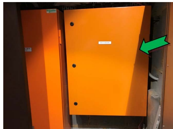
Photo 6. Interior, level 3, switch room, electrical backing board – suspected non asbestos-containing bituminous backing board.
