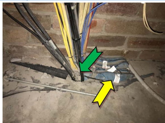
Photo 18. Interior, level 1, comms room, floor, to penetration point – non asbestos-containing mastic sealant and suspected SMF pillow insulation.
