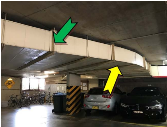
Photo 33. Interior, basement level, air conditioning ductwork – non asbestos-containing mastic sealant and suspected SMF internal insulation.
