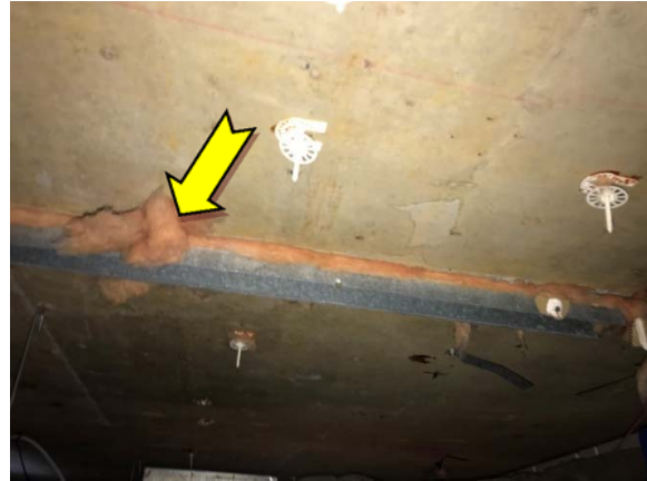
Photo 50. Interior, level 1, ceiling space, to redundant partition supports – suspected SMF insulation material.
