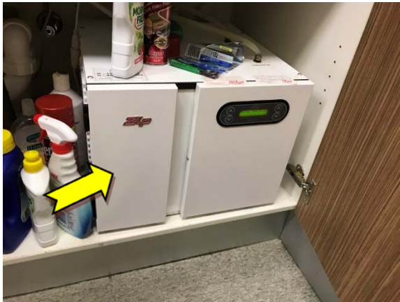
Photo 45. Interior, level 3, kitchen, under sink, hot water heater – suspected SMF internal insulation material.
