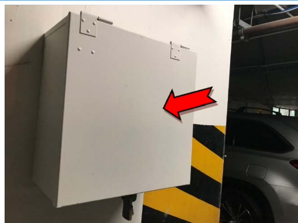
Photo 36. Interior, basement level, west elevation, electrical backing board – suspected asbestos-containing bituminous backing boards.
