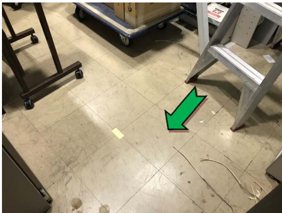
Photo 27. Interior, ground level, IT room, floor coverings – non asbestos-containing vinyl floor tiles.
