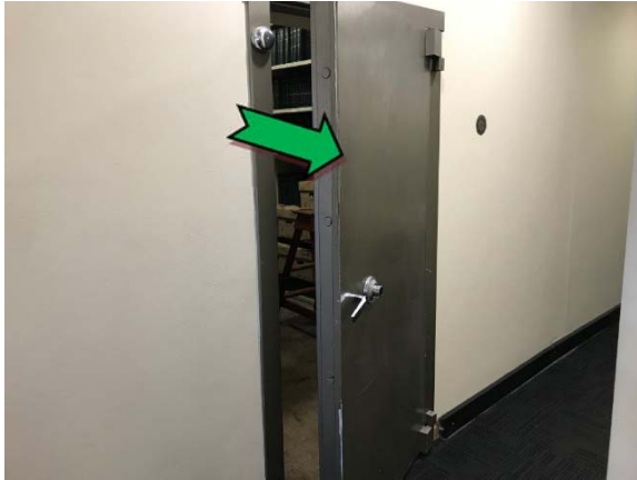
Photo 31. Interior, ground level, strong room, door – suspected asbestos-containing internal insulation material.
