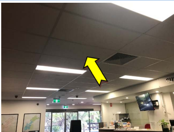
Photo 53. Interior, ground level, throughout, ceiling – suspected SMF compressed ceiling tiles.
