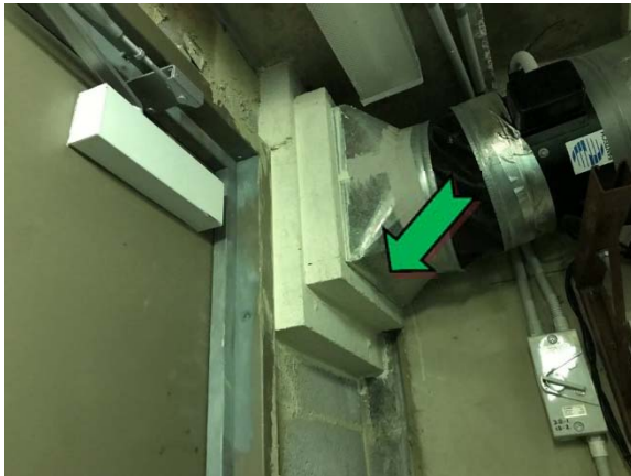
Photo 39. Interior, basement level, pump room, ductwork to wall, infill panel – assumed non asbestos-containing insulating board.
