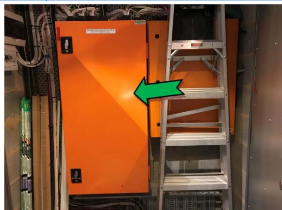
Photo 12. Interior, level 2, switch room, electrical backing board – suspected non asbestos-containing bituminous backing board.
