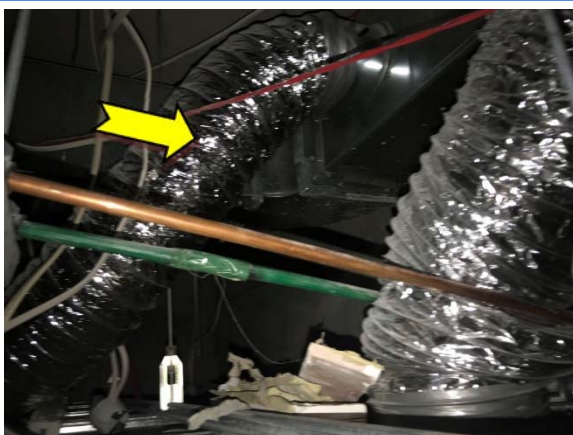
Photo 41. Interior, level 3, ceiling space flexible ductwork – suspected SMF internal insulation material.
