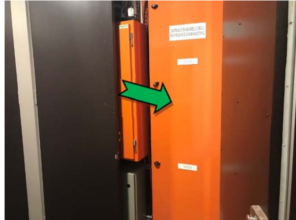
Photo 26. Interior, ground level, switch room, electrical backing board – suspected non asbestos-containing bituminous backing board.
