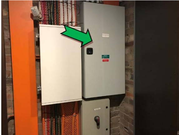
Photo 19. Interior, level 1, switch room, electrical backing board – suspected non asbestos-containing bituminous backing board.
