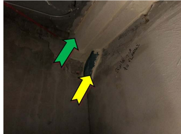
Photo 2. Interior, level 3, training room, ceiling space, to support beams – non asbestos-containing sprayed vermiculite and suspected SMF pillow insulation.
