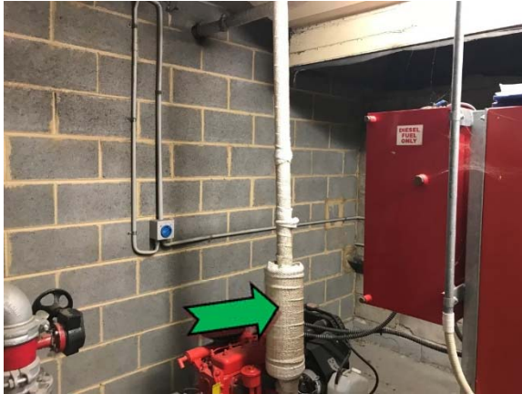
Photo 37. Interior, basement level, pump room, pipe work, to fire pressure pump system – non asbestos-containing woven material.
