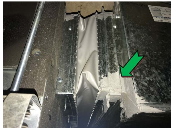
Photo 28. Interior, ground level, ceiling space, air conditioning ductwork – non asbestos-containing mastic sealant.
