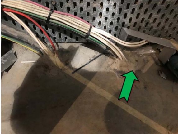
Photo 7. Interior, level 3, switch room, floor, to penetration point – non asbestos-containing mastic sealant.
