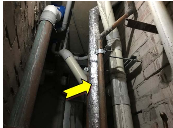
Photo 52. Interior, level 1, men’s toilet, riser cupboard, to pipework – suspected SMF external insulation material.
