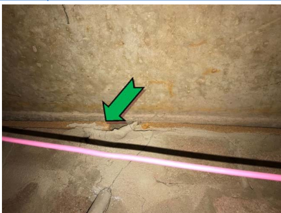
Photo 29. Interior, ground level, corridor to strong room, packing between wall and ceiling – non asbestos-containing fibre cement sheeting.
