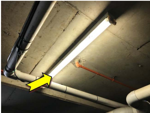
Photo 57. Interior, basement, throughout, single tubed fluorescent light fittings – suspected PCB-containing capacitors.
