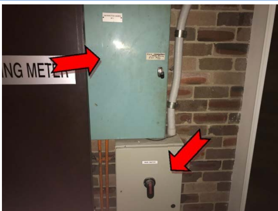
Photo 35. Interior, basement level, opposite lift, electrical backing board – suspected asbestos-containing bituminous backing boards.
