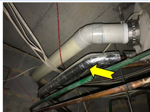
Photo 42. Interior, level 3, west elevation, west elevation, female toilets, ceiling space, to pipework – suspected SMF external insulation material.
