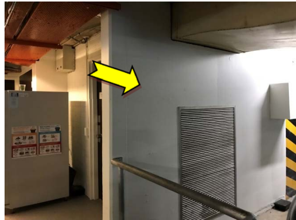
Photo 64. Interior, basement level, wall – lead-containing upper white paint systems.
