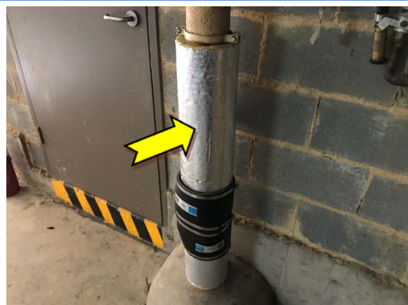
Photo 54. Interior, basement level, to pipework – suspected SMF insulation material.
