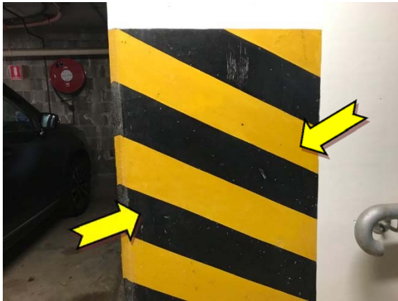
Photo 63. Interior, basement level, column – lead-containing yellow upper paint system and suspected lead-containing black upper paint systems.
