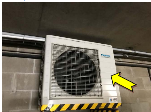
Photo 66. Interior, basement level, air conditioning unit – suspected ODS-containing unknown refrigerant
