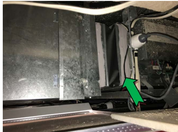
Photo 10. Interior, level 3, throughout, ceiling space, air conditioning ductwork – suspected non asbestos-containing mastic sealant and suspected SMF internal insulation.
