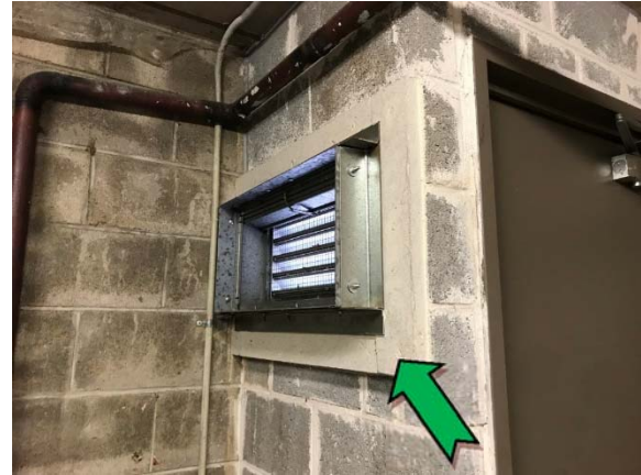
Photo 38. Interior, basement level, pump room, south elevation, infill panels – assumed non asbestos-containing insulating board.
