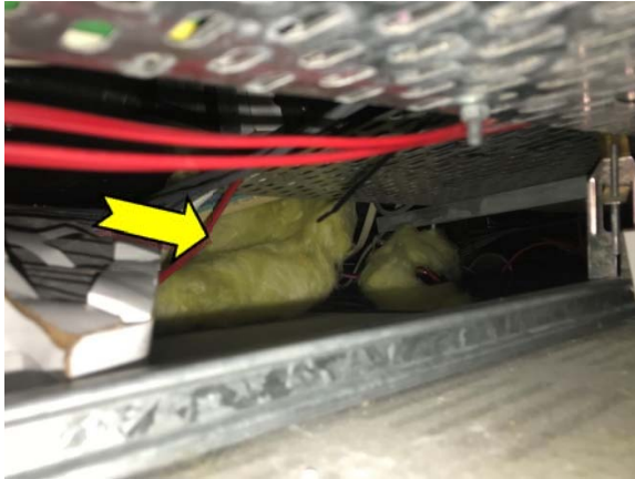
Photo 43. Interior, level 3, ceiling space, throughout – suspected SMF insulating batts.
