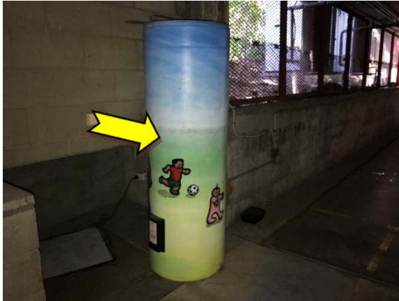
Photo 55. Interior, basement level, west elevation, hot water heater – suspected SMF internal insulation material.
